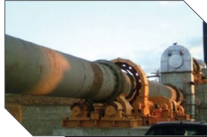
Kalsine Manyezit Tesisi Calcined Magnesite Plant
