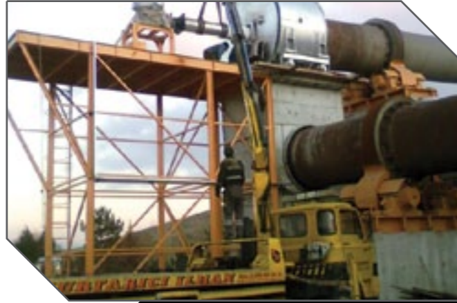
Kalsine Manyezit Fırın Brülörü Calcined Magnesite Rotary Kiln Burner
